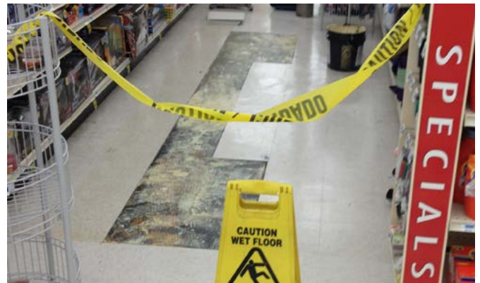
... and causes downtime and high repair costs
